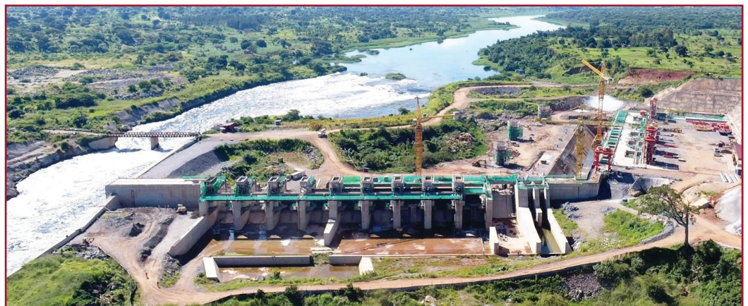
Right: The Karuma Hydroelectric Power Station - under construction in Uganda - will generate 600 MW of additional power to the National Grid.
